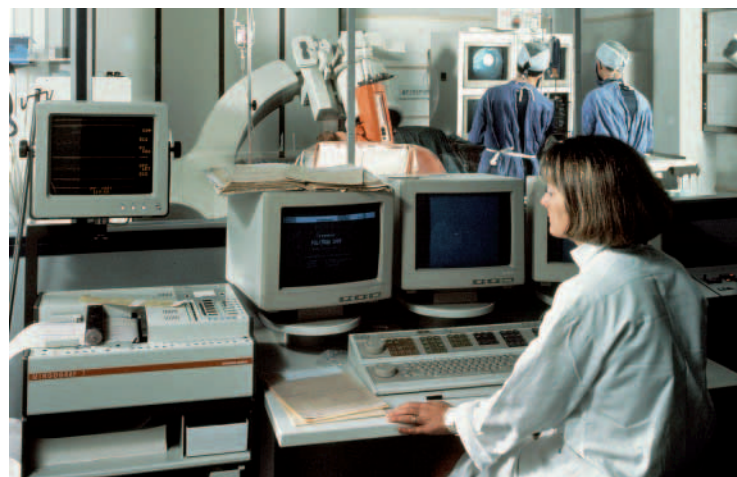
Room and equipment for operating radiology
