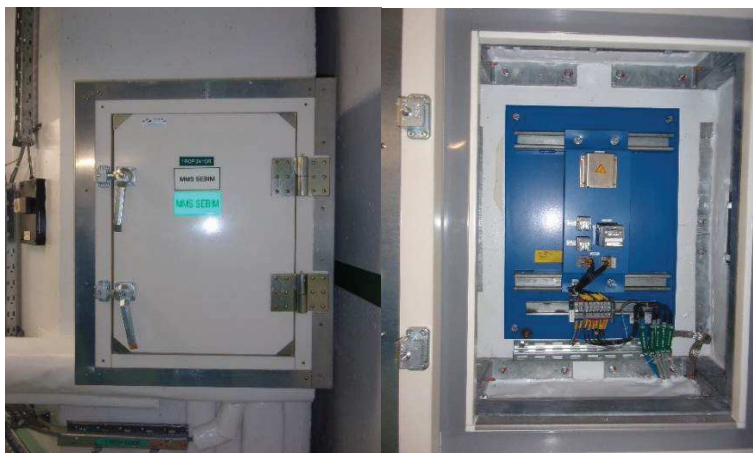
Installed Electrical Cabinet for opening of the pressurizer relief valves.
