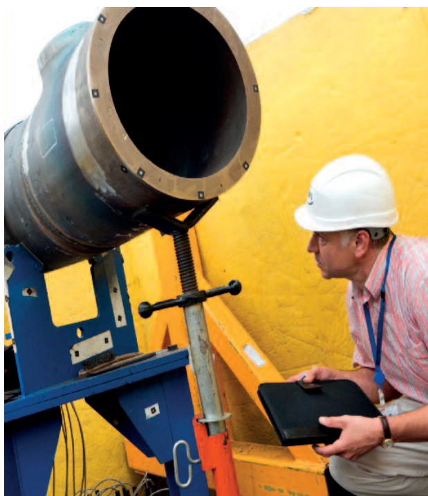
ASN check on prefabrication of a secondary system pipe during replacement of steam generators at Fessenheim 2 – September 2011
