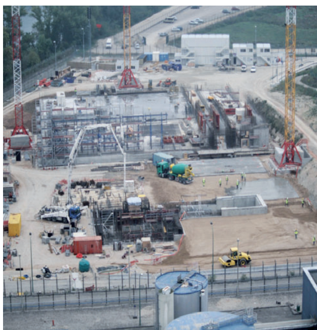
Construction progress on the waste packaging and interim storage site (ICEDA) at Bugey – October 2010
