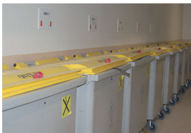
Solid waste containers in the interim storage area of the nuclear medicine department – Nancy CHU – December 2010
