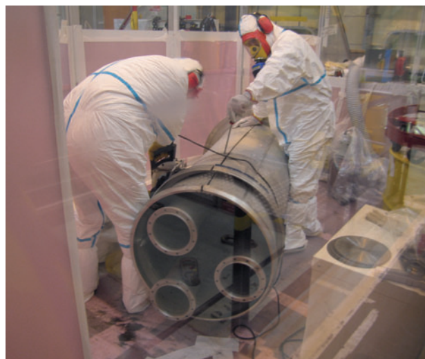
Cutting operation on an item of equipment of the PHEBUS experimental reactor at Cadarache
