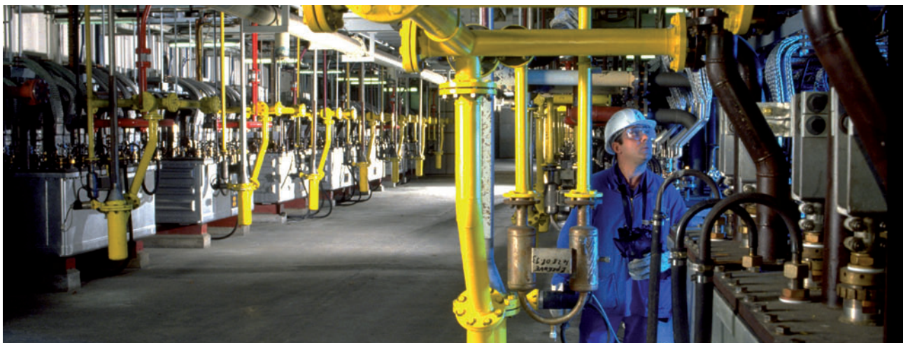
Fluorine electrolysis cells. COMURHEX Pierrelatte plant for converting UF 4 to UF 6 , Tricastin site
