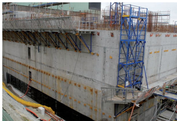
Construction of an extension to the fission product interim storage hall (CSD-V)
