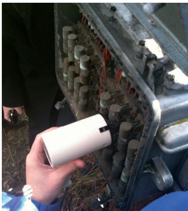
Interior of box containing radioactive surge suppressors - radioactivity measurement in progress
