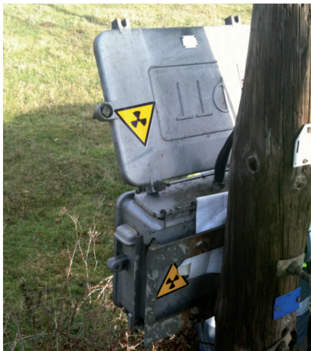
Box containing radioactive surge suppressors
