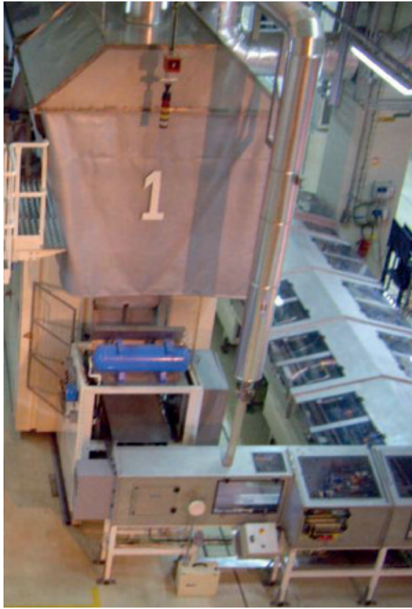
New sintering furnace for the uranium pellets production line in the FBFC plant in Romans-sur-Isère (Drôme département)
