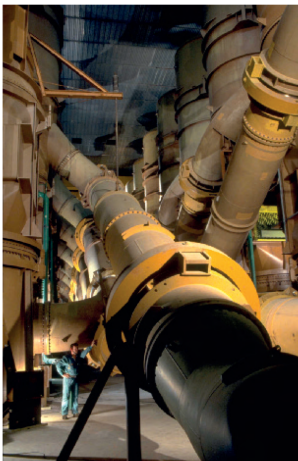
Decommissioning of Eurodif on the Tricastin site (Drôme département) will lead to the decommissioning of about 150,000 tons of steel
