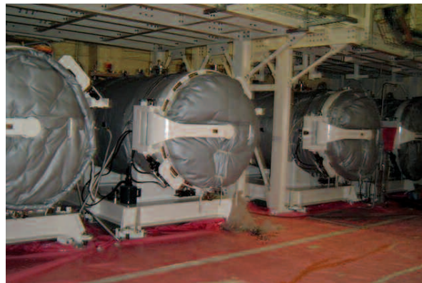
FBFC – New autoclaves at Romans-sur-Isère
