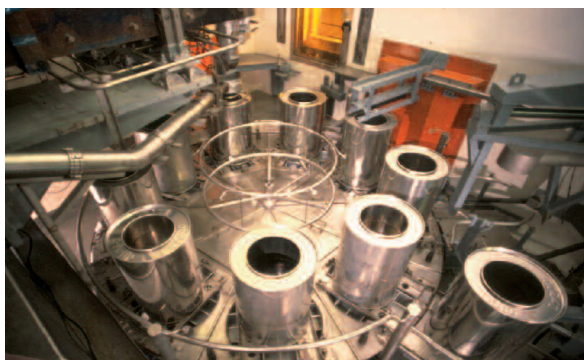
AREVA NC La Hague – Drum filling equipment in the STE3 station
