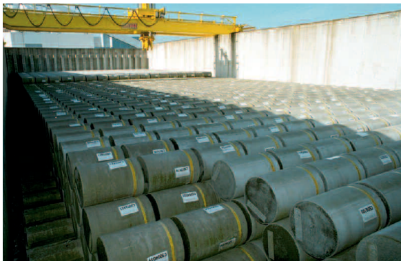
AREVA NC La Hague – Interim storage of waste drums in the ADT facility
