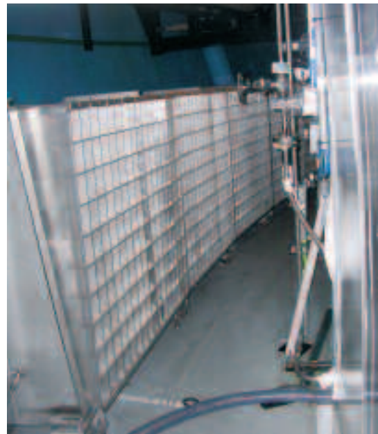
New sumps installed by EDF in 2005
