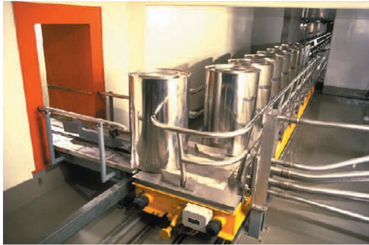
La Hague – STE3: automatic transfer of bitumen containers
