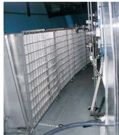
New sumps installed by EDF in 2005
