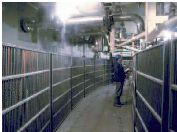
N4 plant series reactor sumps
