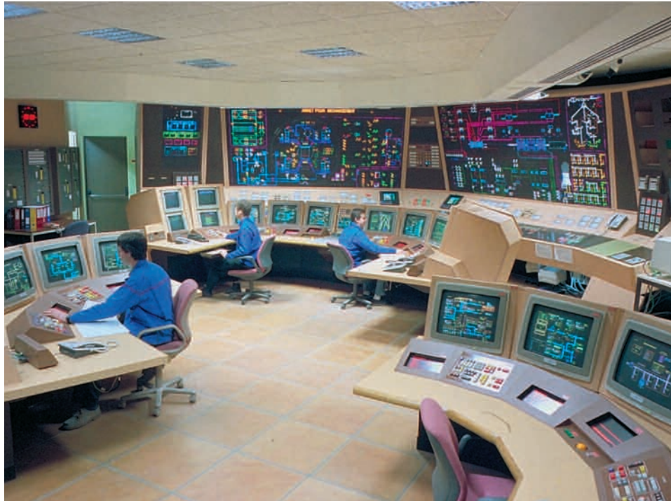
N4 reactor control room
