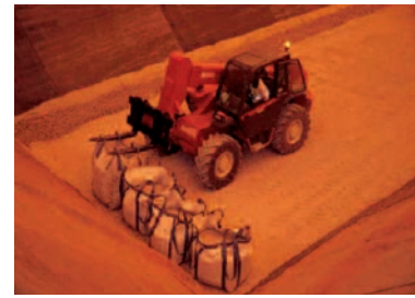
ANDRA – receipt of packages at the Morvilliers very low level waste repository
