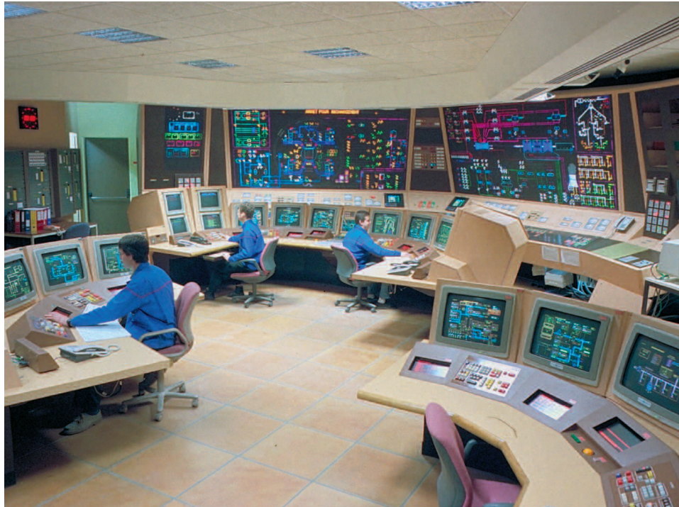
N4 reactor control room
