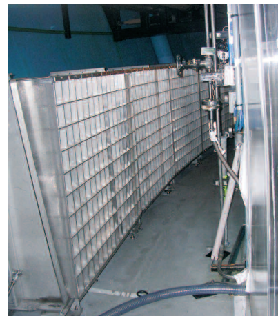
New sumps installed by EDF in 2005
