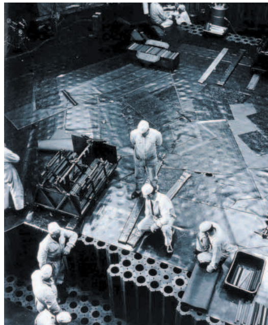
Graphite stack in a gas-graphite Uranium reactor
